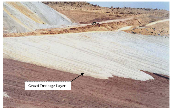
Fig. 12. Site view of the heap structure 2 along with construction of the gravelly drainage layer at Sarcheshmeh copper mine.
